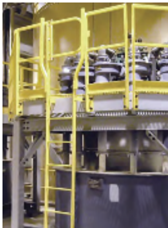
Raised platform with protected guardrail.
